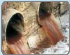
Poor Industrial Waste Disposal
